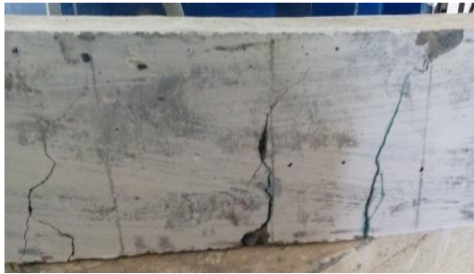
fig 2. Crack pattern of specimen
